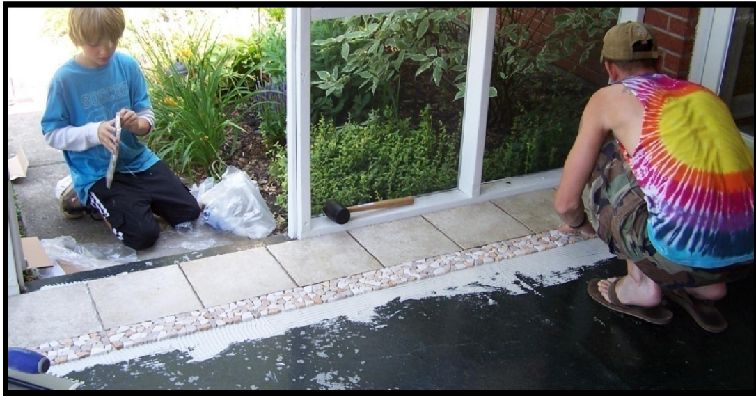
Allen models patience and respect while encouraging Trae to carefully spread grout and match the tiles on our front porch.
